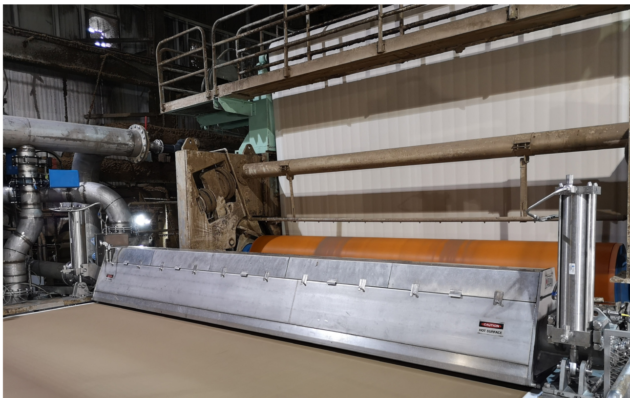
SSV in operation without any visible steam spillage
